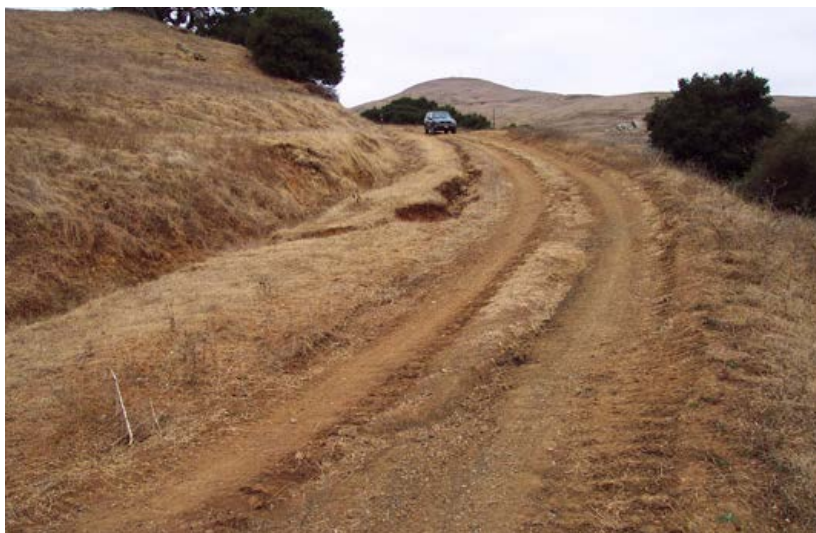
A RUTTED AND GULLIED ROAD, BEFORE TREATMENT
