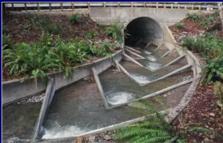
Full Width "Vortex" Pool-and-Chute Fishway
