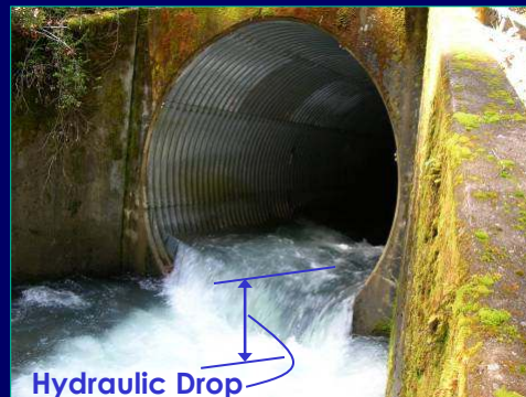
High Fish Passage Flow (excessive hydraulic drop)
