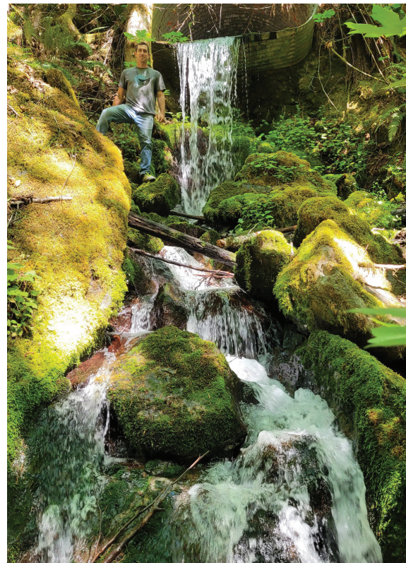
Rapid assessment of perched culvert in the Smith River watershed, 2021.
