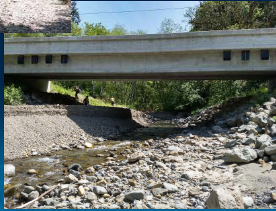
Little Mill Creek Bridge Depositional Bar from River Backwatering – adequate capacity
