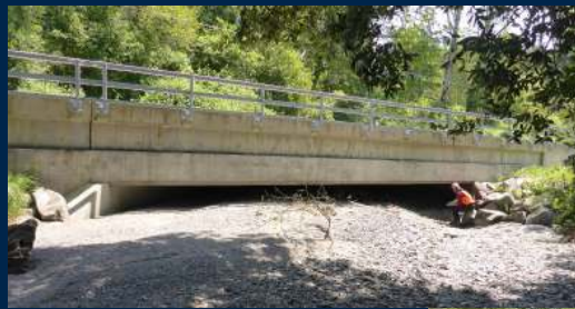
Sultan Creek Bridge Influenced by Debris Jamming from High Flow Backwatering by Smith River – inadequate capacity
