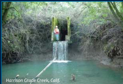
Harrison Grade Creek, Calif. Perched Culverts
