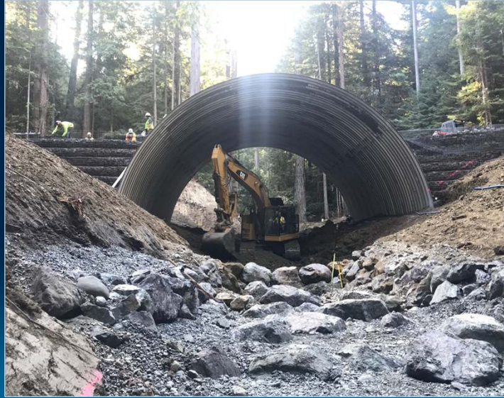
Upper Noyo River Crossing: 3.6% Boulder Step Pool Channel thru 50-ft span arch
