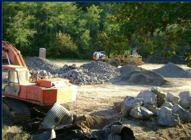
3. Stockpile ESM onsite. Within a small section of channel, place material in correct proportions and mix with excavator bucket ...
